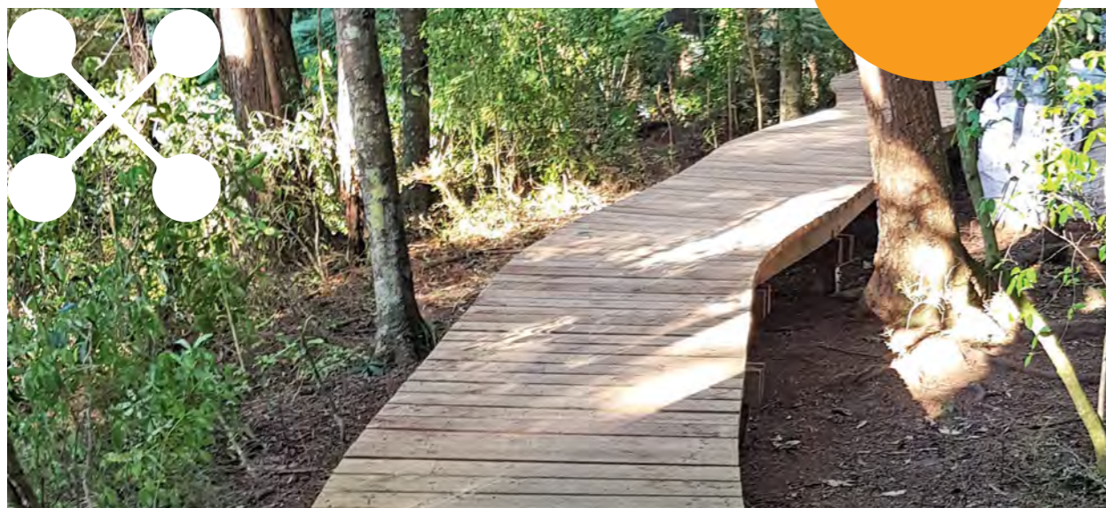
The new boardwalk in Albany is built around large trees to protect vulnerable roots.
