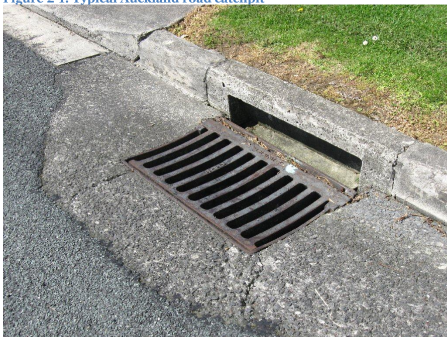
Figure 2-1: Typical Auckland road catchpit
